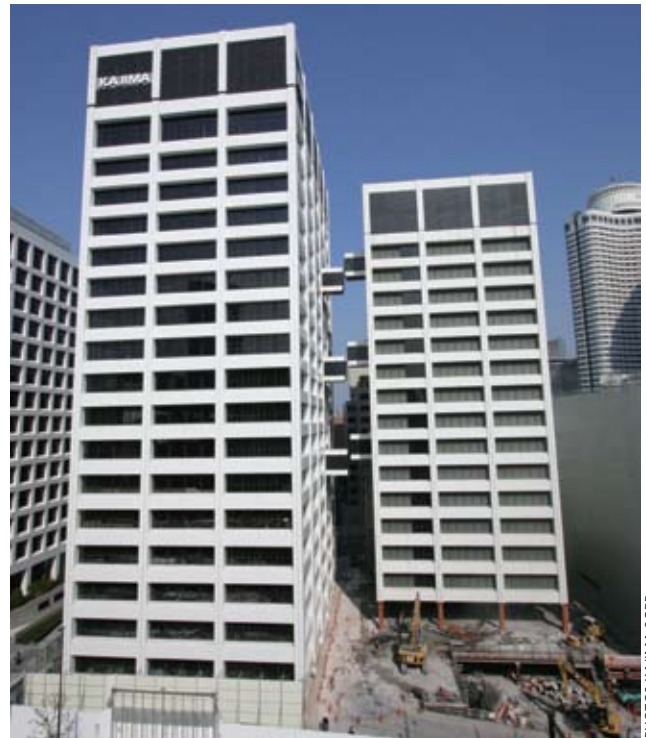
Kajima Corp. is using its “Cut and Down” method on their former HQ buildings. PHOTOS: KAJIMA CORP.
